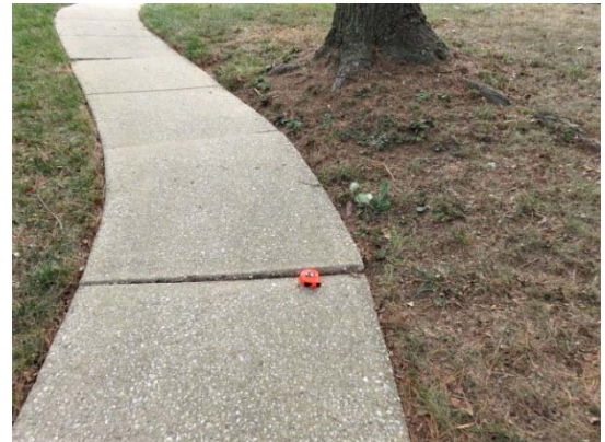
Concrete heaved by tree roots, trip hazard
