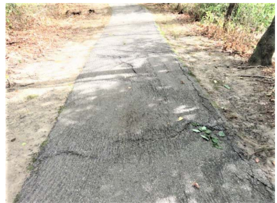
Typical path raveling, cracking and ageing conditions
