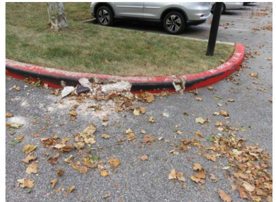
Curb damaged by vehicle traffic
