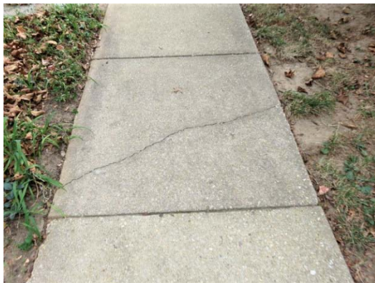
Typical cracking condition
