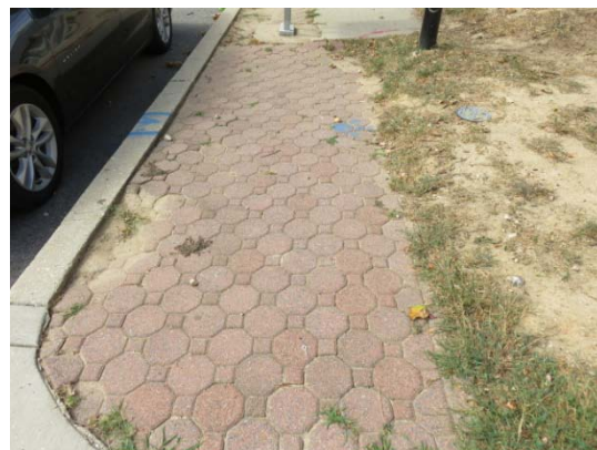
Pavers at mailbox area settled below curb line
