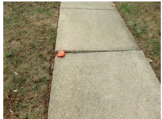
Concrete section settled, trip hazard
