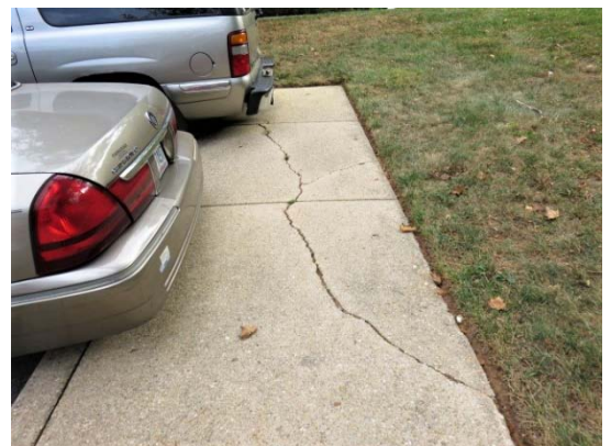
Typical monolithic curb / sidewalk cracking
