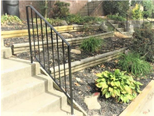
Typical 3" X 5" retaining wall, displaced & leaning
