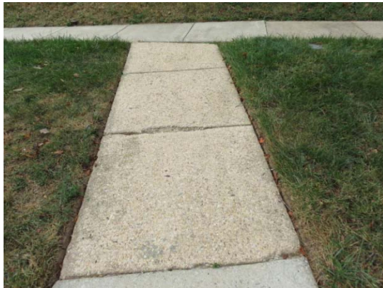
Typical scaling condition
