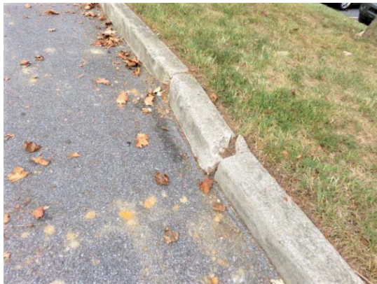
Broken barrier curb section
